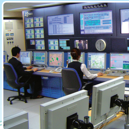
VICS Center (Monitor Room)
